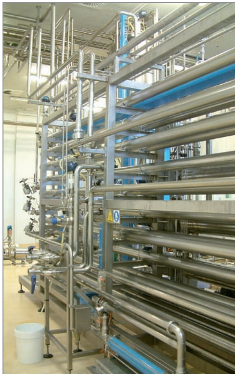
A section of the new production line
