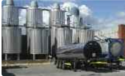
The road tanker bay at Dundalk.
