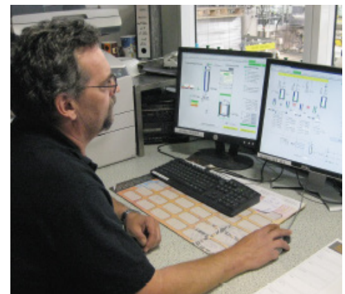
Within six months, the previous control system was replaced by the modern Plant iT V8 process control system
