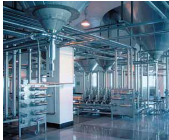
Fermentation cellar of the Yanjing Beer Group Beijing/China
